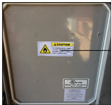
INSIDE OF ELECTRICAL BOX
